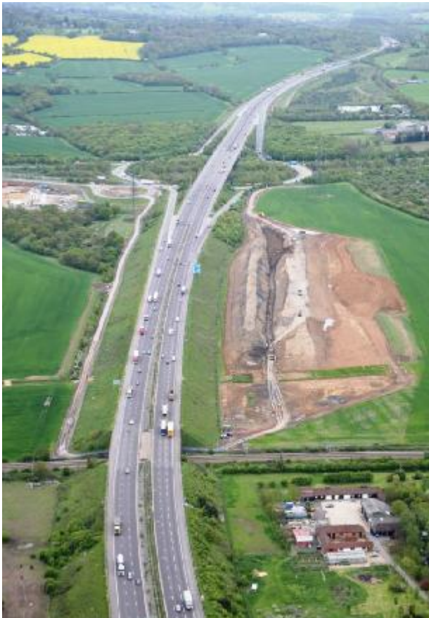
Upminster Bund under construction. This bund will finally be 4m above the carriageway and is to protect the residents of Cranham from the M25.
